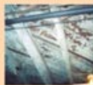
1. Mold Damage on Floor Joists
